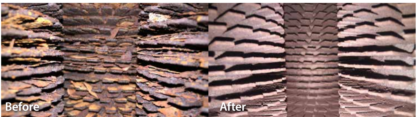
Sonic blasting inside the McWilliams HRSG proved effective in cleaning debris from boiler pipes.
